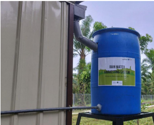
Figure 4: Rain Water Harvesting System. Used to collect and store rainwater for various non-potable applications. The stored water can be used for garden irrigation, washing outdoor areas and cleaning tools. This system helps conserve municipal water and provides an eco-friendly solution for small agricultural needs.
