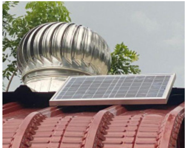
Figure 5: Solar System and Wind Turbine Ventilation. Solar panels generate renewable electricity for lighting in the cabin. Wind turbine ventilators passively remove hot and stale air from the cabin, increasing airflow and keeping the interior cooler without using electricity. These work together to improve energy efficiency and ventilation.
